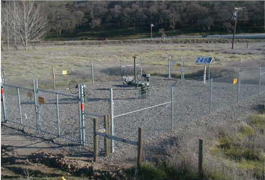
Photo 1: Typical fenced aboveground pipeline valve lot with aboveground portions of valves
