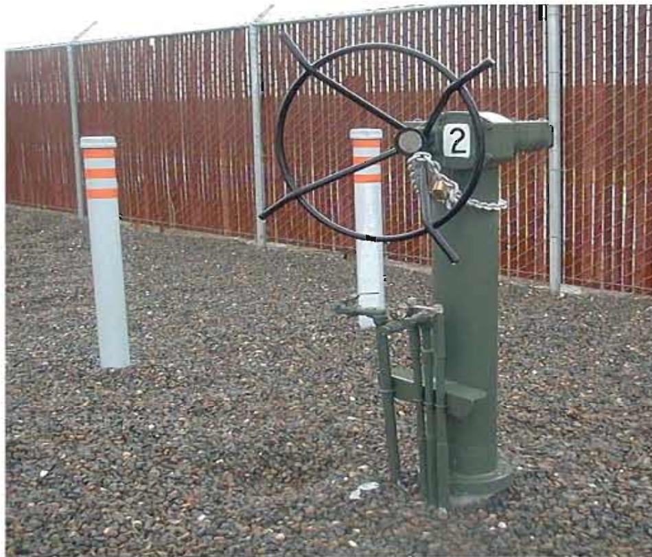
Photo 2: Typical aboveground portion of pipeline valve
